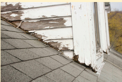
Third-floor windows and dormers need replacement
